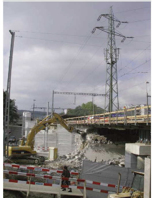
During demolition of parts of the foundation of the power line pylon, the monitoring system was used to detect 3D deformations and the resulting change in tilt.
