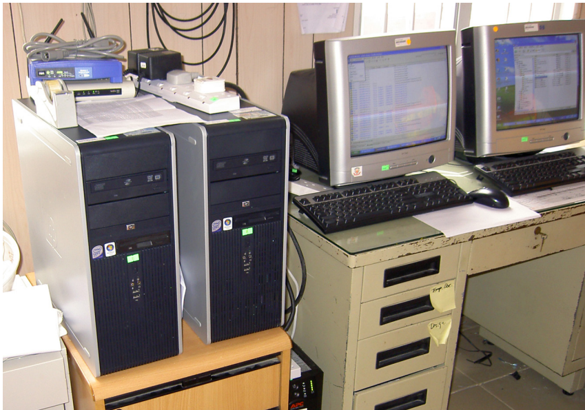
Control Center of the Monitoring System
