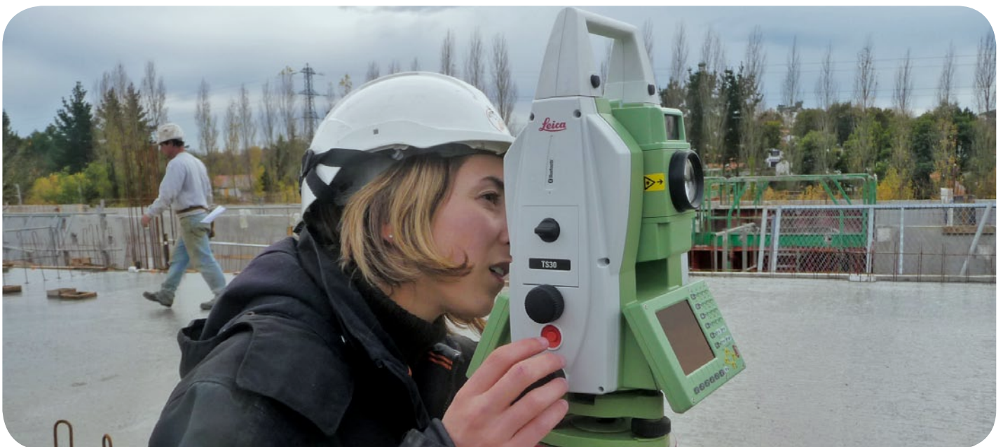
■ Precision stakeout of the curtain wall façades: surveying engineer Julie Deléglise with the Leica TS30.
