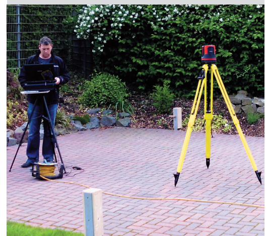
The Leica 3D Disto records exactly the shapes of the area and marks the assembly points.
