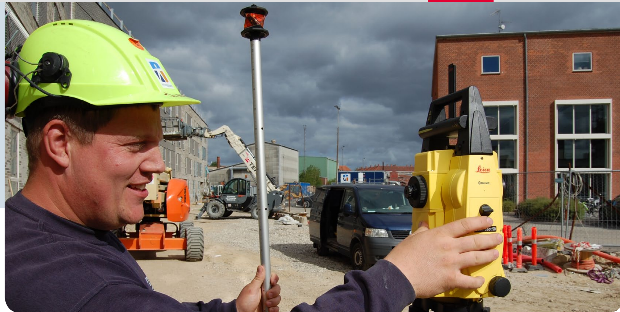
■ Jonas Nielsen finishing a subcontractor job preparing the terrain for a large house-building project.
