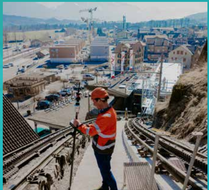
Fabian Nebel, Head of Construction and Engineering Surveying at Trigonet AG uses the Leica AP20 AutoPole to measure on the construction site of the steepest cog rail in the world, the Pilatus Cog Rail by Lucerne, Switzerland.
