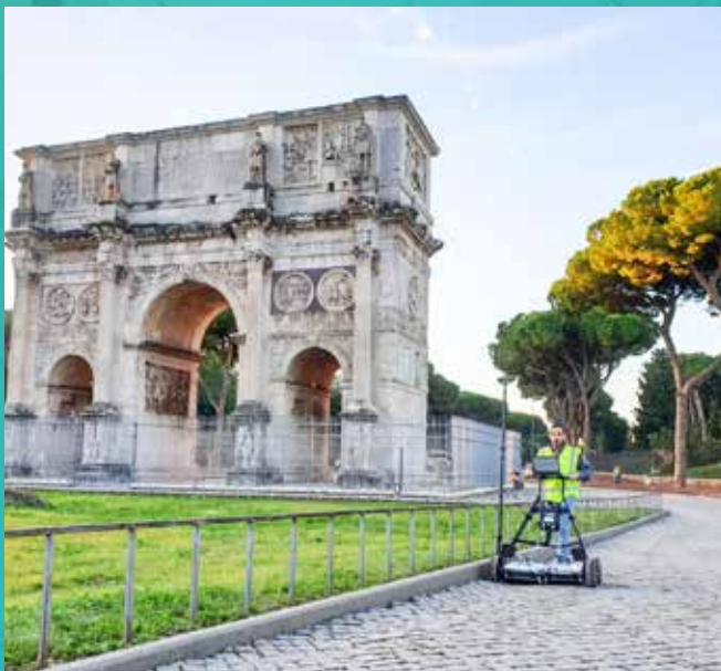
ACEA company is performing extensive utility detection in the centre of Rome with the all-in-one specialised GPR system RIS MF Hi-Mod. Photo by BOVIAR srl.
